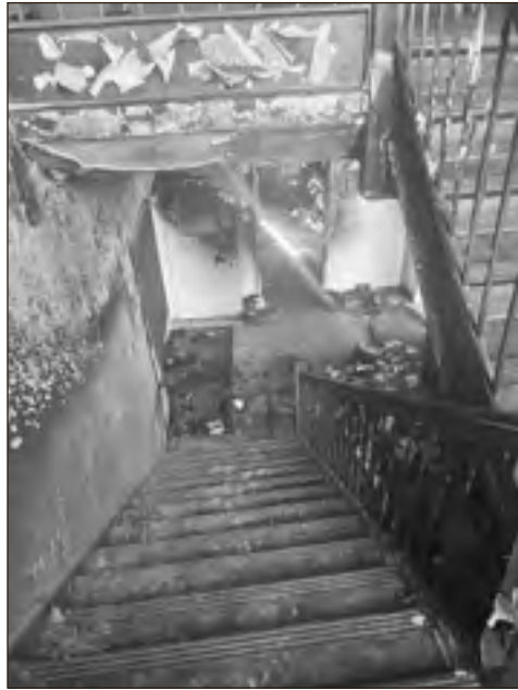
The damage was so intense it will likely take until May, maybe longer, before it becomes operable once more.
